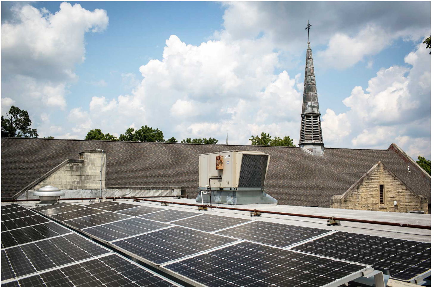
Solar panels line the roof of Downey Avenue Christian Church in Indianapolis.
